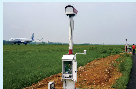
DRISHTI at Lucknow Airport, Nov. 2015
