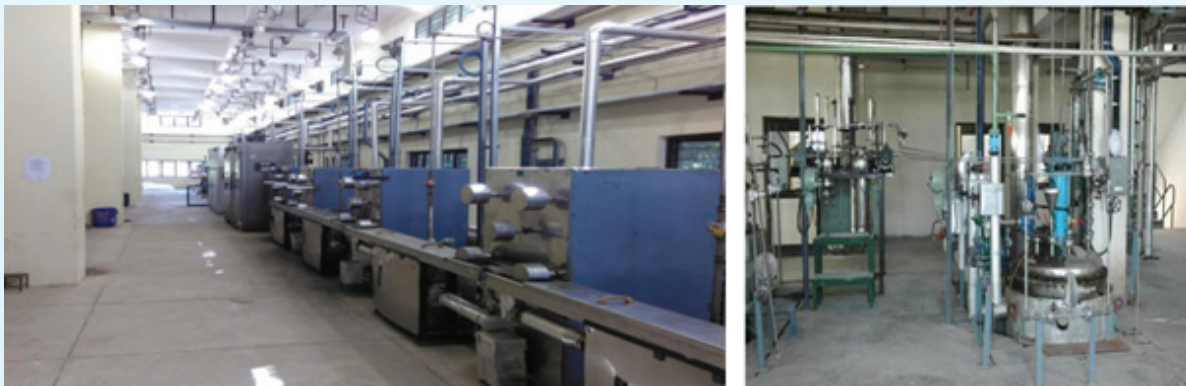
Carbon fibre plant at NAL
